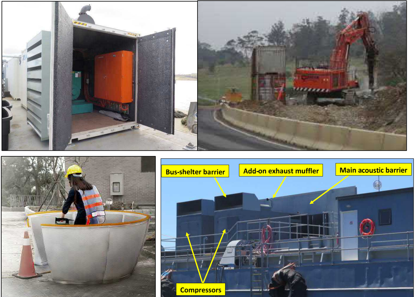
Figure 2 Top left. A 550 kVA generator inside a shipping container lined with acoustic material. Two high performance acoustic louvres provided ventilation, and on top is a custom-designed muffler.
